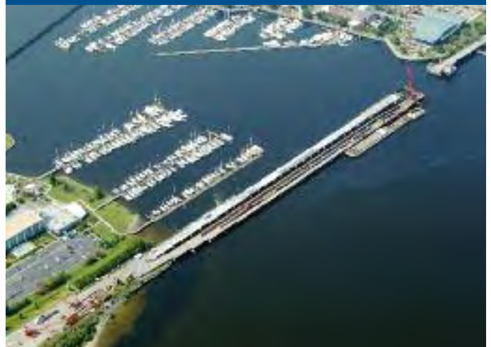
Good progress was made on the contract to replace the Trent River Bridge in North Carolina.
