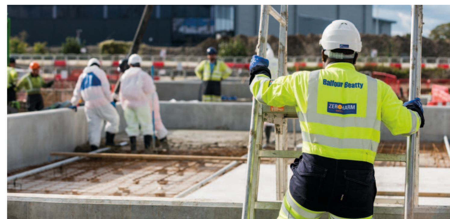
Littlebrook Substation, Kent
