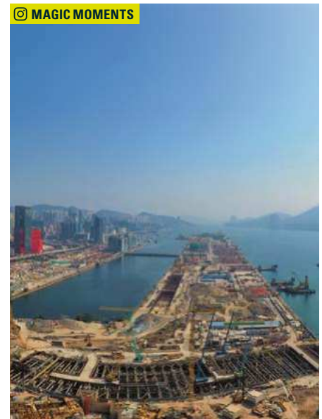
Hong Kong: Central Kowloon Route - Kai Tak West, Highways Department, HKSAR Government. Photo credit: Lunggy Fung
