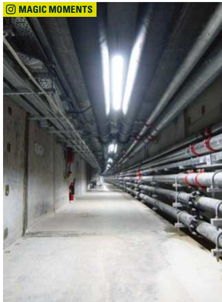
Hong Kong: Central Kowloon Route - buildings, mechanical and electrical works, Highways Department, HKSAR Government. Photo Credit: Lee Ho Hang
