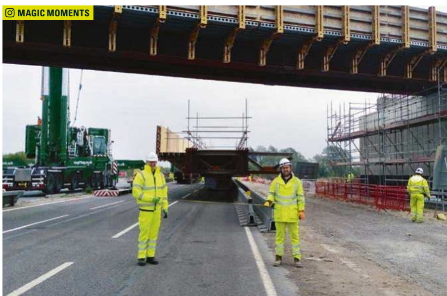
UK: The installation of a new bridge at Marsh Lane on the M4, Highways England. Photo credit: Leo Quinn
