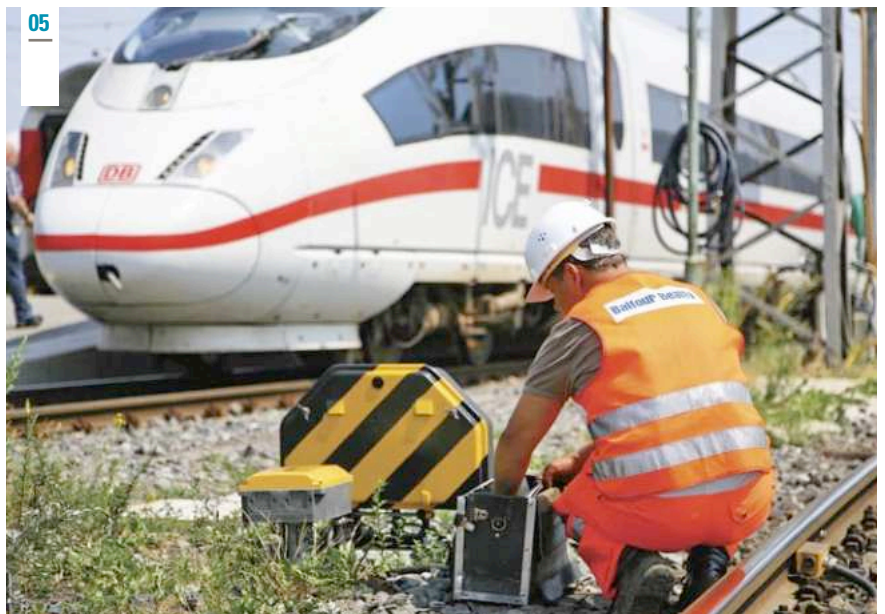
05 Rail electrification, Dortmund – Balfour Beatty Rail Germany
