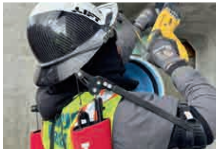
ABOVE Exoskeleton in use on the Harkers Island Bridge replacement project in North Carolina.
